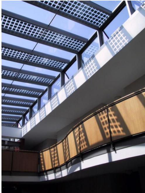
Figure 18. The BIPV skylight comprising an alternating pattern of glass and BIPV modules
