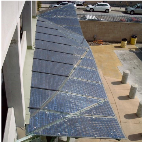
Figure 10. The BIPV system comprising of 28 different BIPV modules
