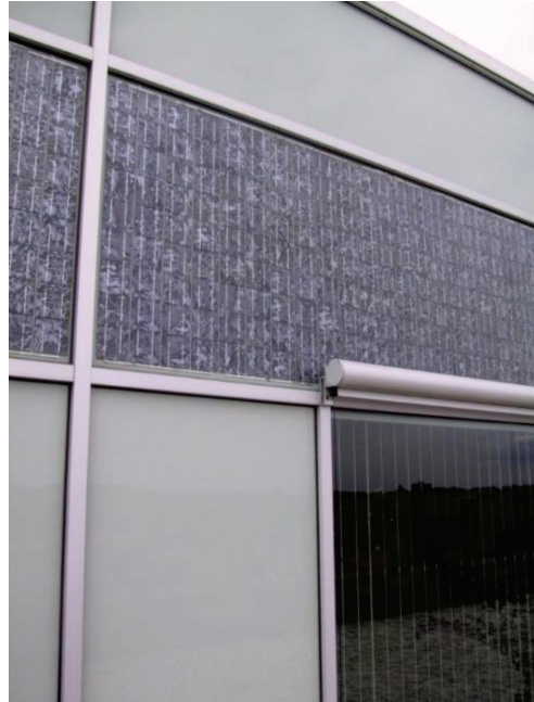
Figure 20. Exterior shading blinds installed during building renovation not considering the shading of the adjacent BIPV modules
