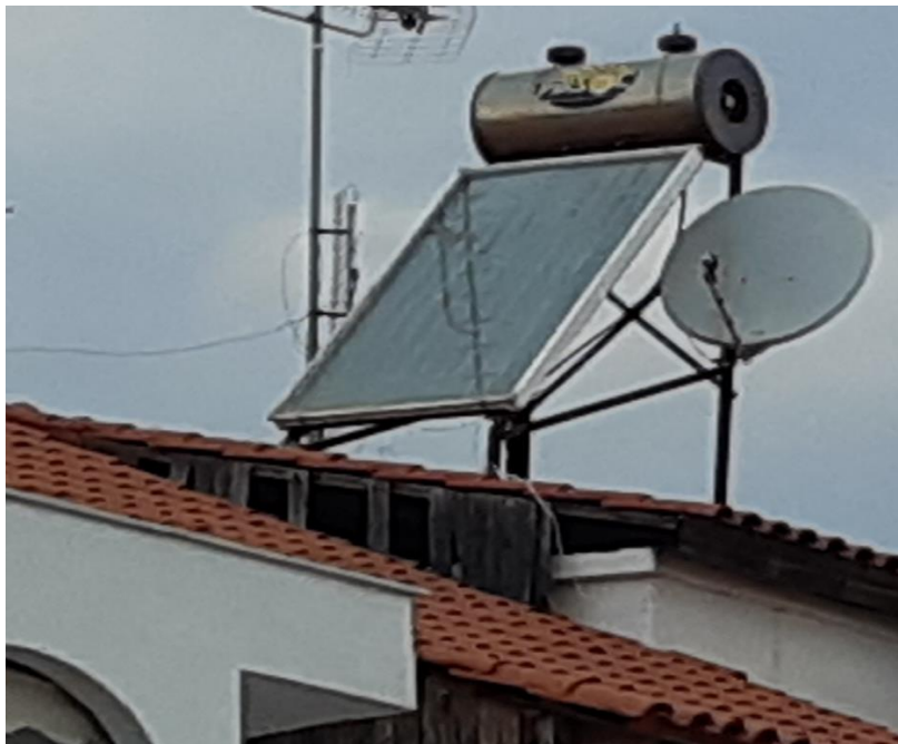
Figure 7. Solar collectors for water heating
